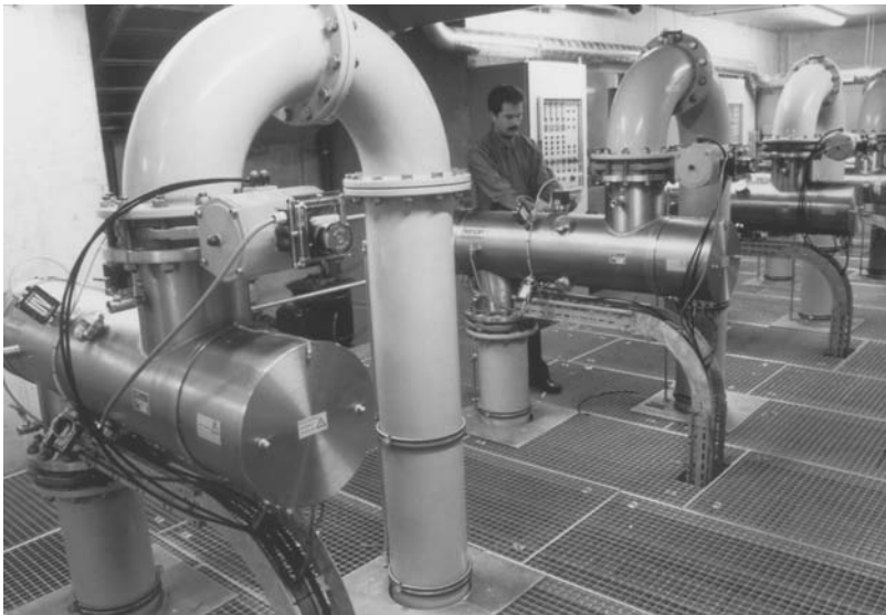
FIGURE 89 Roosteren, the Netherlands: 1000 to 1600 m 3 /h at T_{10} 97\% for disinfection of groundwater; 20 Berson 2500 (medium-pressure Hg with multiple emission wavelengths) installed in four parallel reactors.
