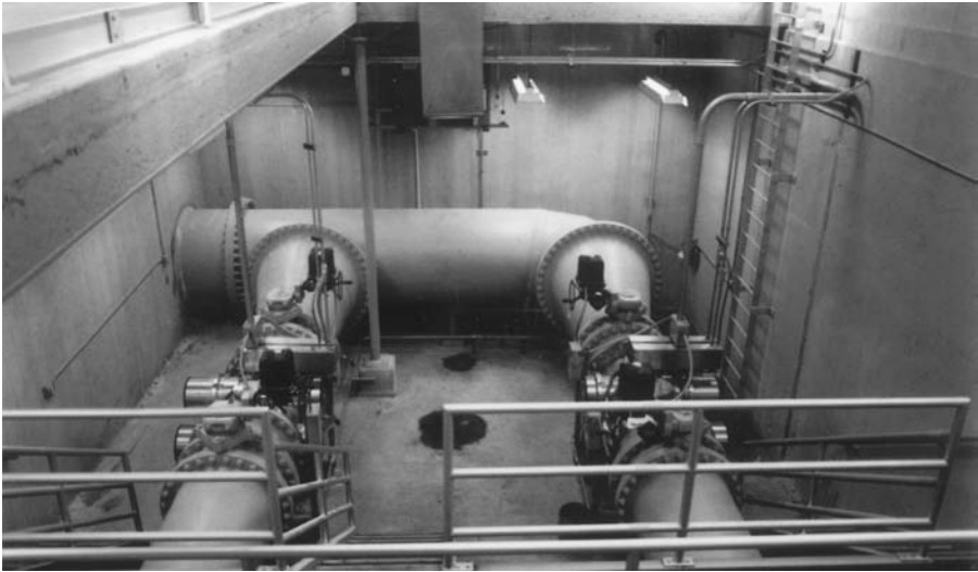
FIGURE 103 Plant at Newcastle, Indiana. This plant (designed by Berson) can treat 1570 \text{ m}^3/\text{h} of a treated effluent with a transmittance of T_{10\%} of 60. Two chambers are each equipped by 24 lamps mounted in the transverse mode. The equipment has been installed in preexisting buildings.
