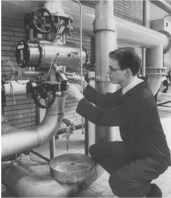
FIGURE 88 Zwijndrecht, the Netherlands: disinfection of potable water from bank-filtered water; T_{10} = 85\% ; four units of four Hg medium-pressure lamps each emitting multiple UV wavelengths.
